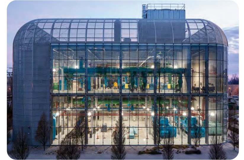
University of Chicago South Campus Plant
